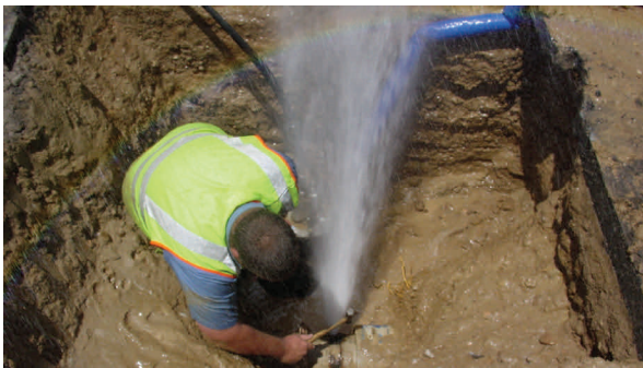
Water Gushing...Emergency - Yes
